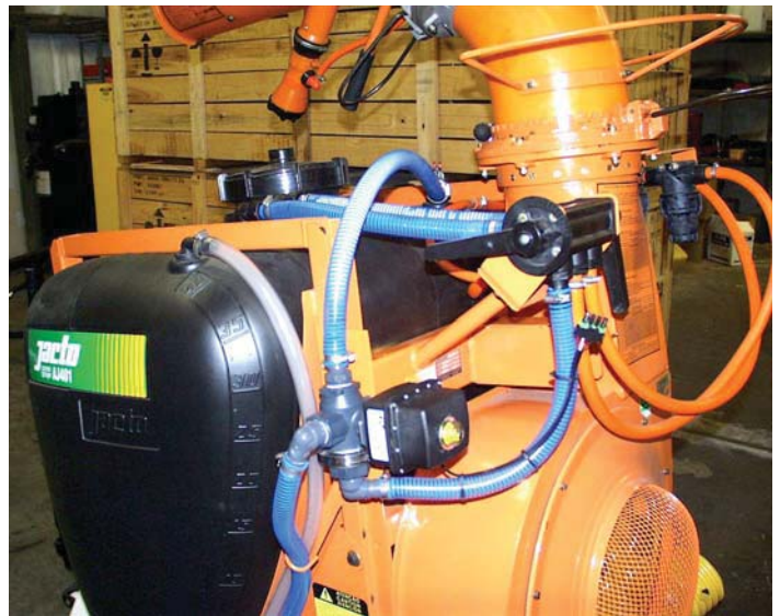
Electric valve installed with all hoses attached
