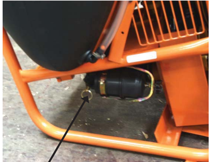
Filter shut off
